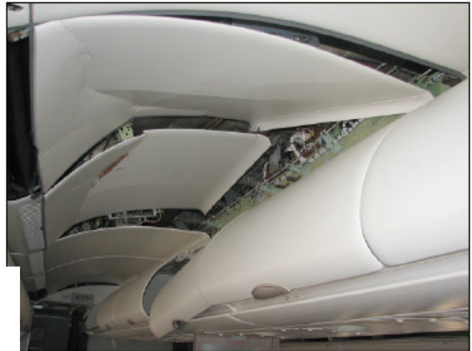
Figure 50: Example of damage to the ceiling panels in the aisle (rear section)
